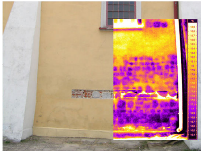
Figure 6.8: Visual light photo of a wall with overlaid thermal image – thermal pattern revealing subsurface structure is due to solar loading
